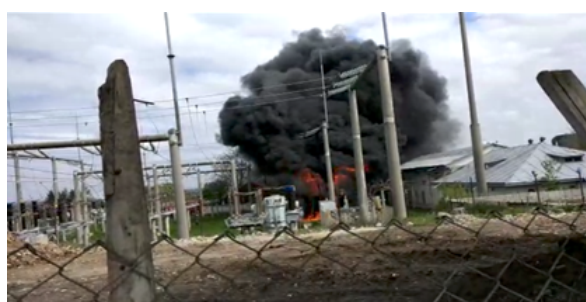
Fig. 2. Explosion and burning of several transformers in Botoani - RO [3] (2017)
