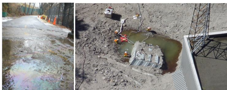
Fig. 1. Washington DC (USA) 2011- from an disabled transformer about 21.000 liters of mineral oil was spilled on the soil and in Potomac River [2]
